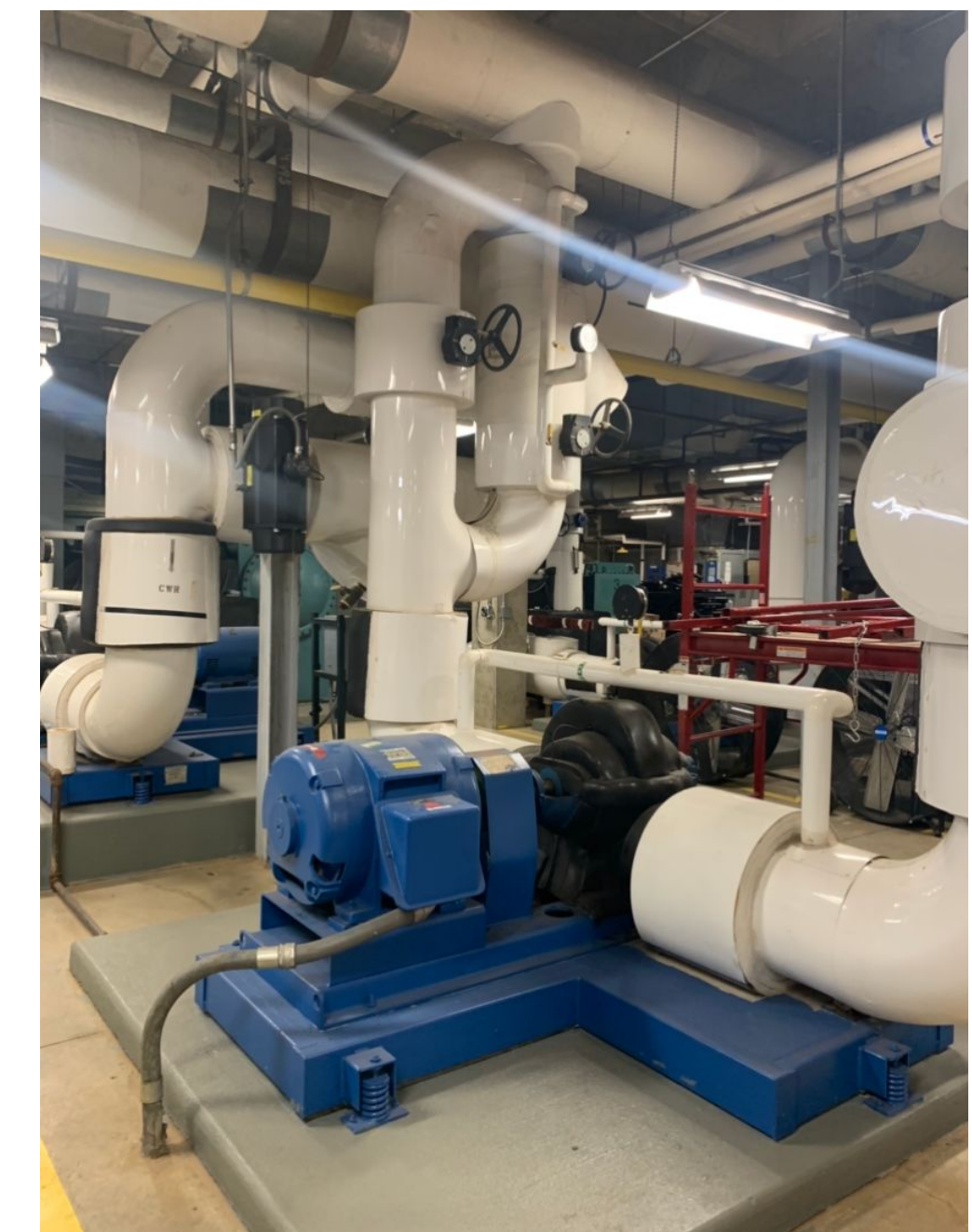
Tour of utility system at the Schottenstein Center
