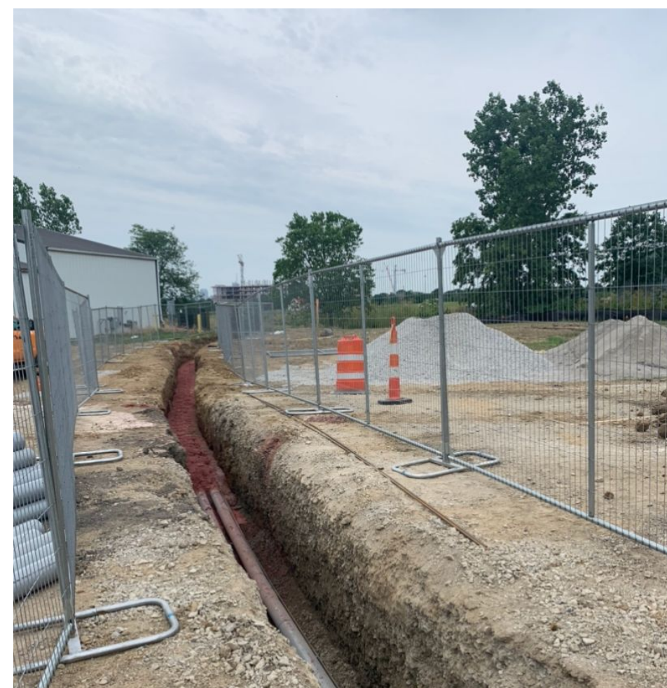
One of the main projects of the program manager that I worked with this summer was installing utility lines at the new Controlled Environment Food Production Research Complex. These pictures were taken throughout the process at the site inspections that I attended.
